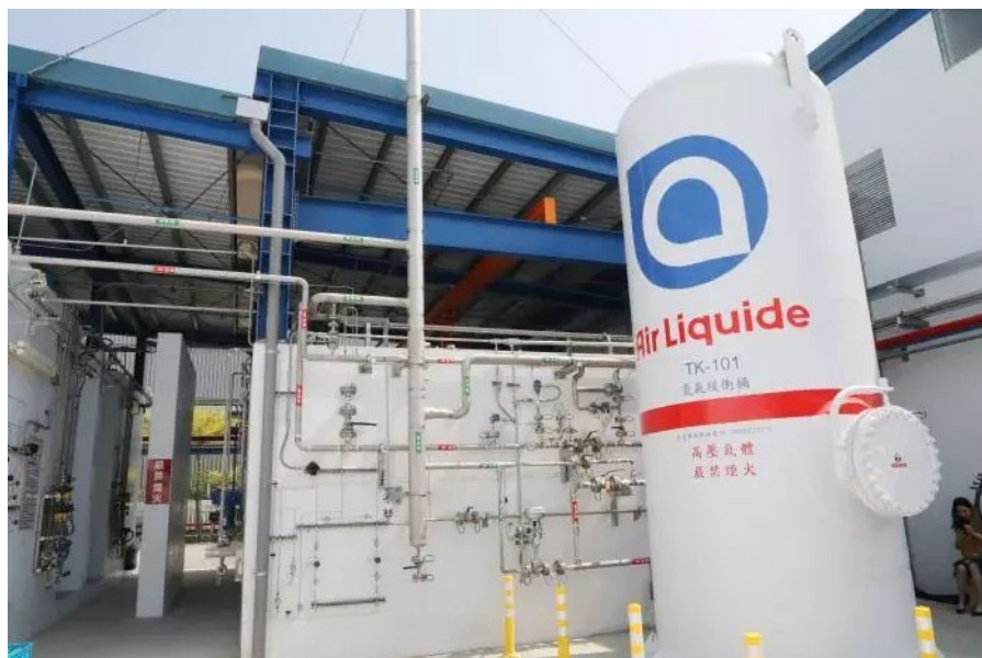
Figure 19. 25 MW low carbon water electrolysis plant of Air Liquide Far Eastern Company
